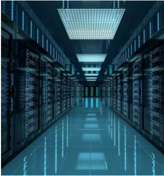
Data Center Solutions
